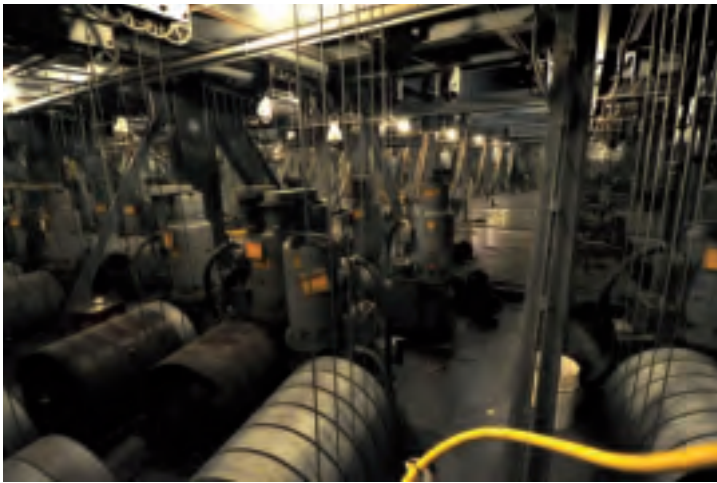
Pipe Motor Grid Iron: 120 feet above the deck
