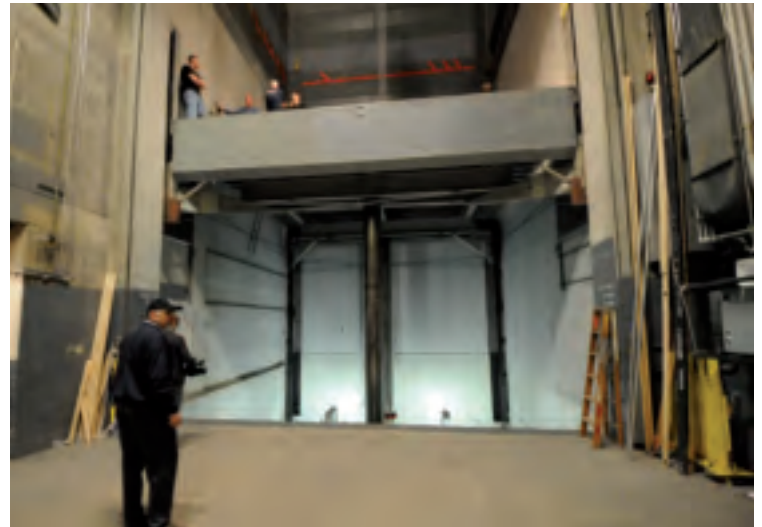
The Hydraulic Stage Scenery Lift From "C" Level (basement) to the Great Stage
