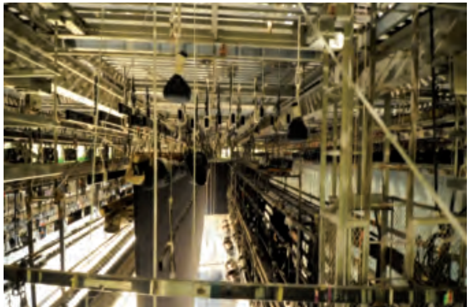
Underside of the Grid Iron with a Light Bridge on the Lower Right.
